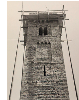
The tower during the restoration work in 1945. A concrete crown was inserted to maintain its structural integrity.
