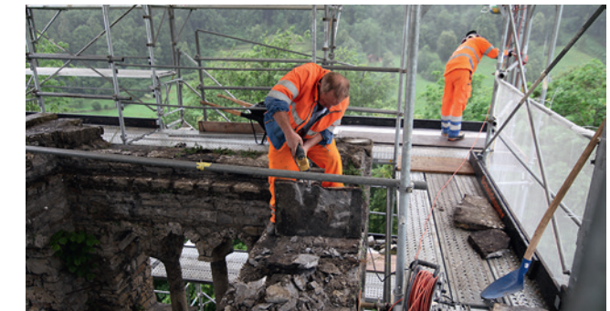
Craftsmen at work on the upper tower terminal during the restoration in summer 2015.
